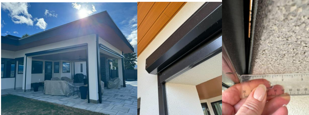
Photo 7. Motorized Talus roll down blinds with housing, not on a timer. Although there are 3 blinds, bats only use the North-facing one. They have seen several bats per year since 2022, sometimes in pairs. Bats roost behind the screen in the 1/2" gap against the stucco. They do not get injured there.
