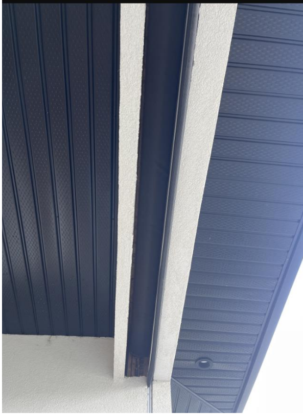
Photo 5. Motorized Phantom screen, not on a timer. This awning faces east and is shading a deck. Reported finding 5 dead dried up bats in between the layers of the roller screen. Homeowner assumes the bats got stuck between the layers of the roller screen when rolling up the shade. The gap is 6" wide.
