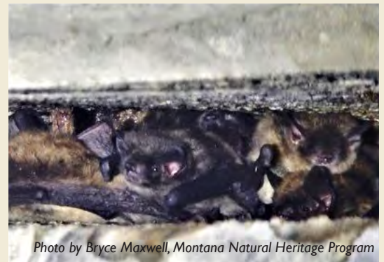
Bats roosting in an expansion joint of a concrete bridge.
